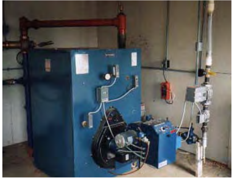
Photo: Moser M, RCM Digesters, Inc.
