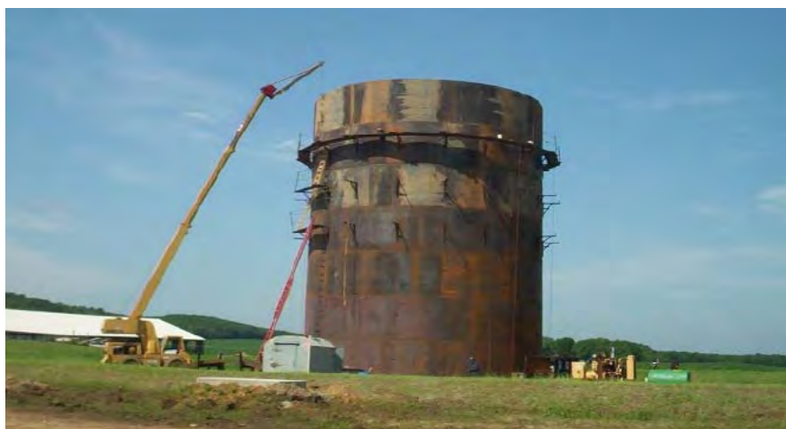
Photo: Eastman D, Microgy Cogeneration Systems
